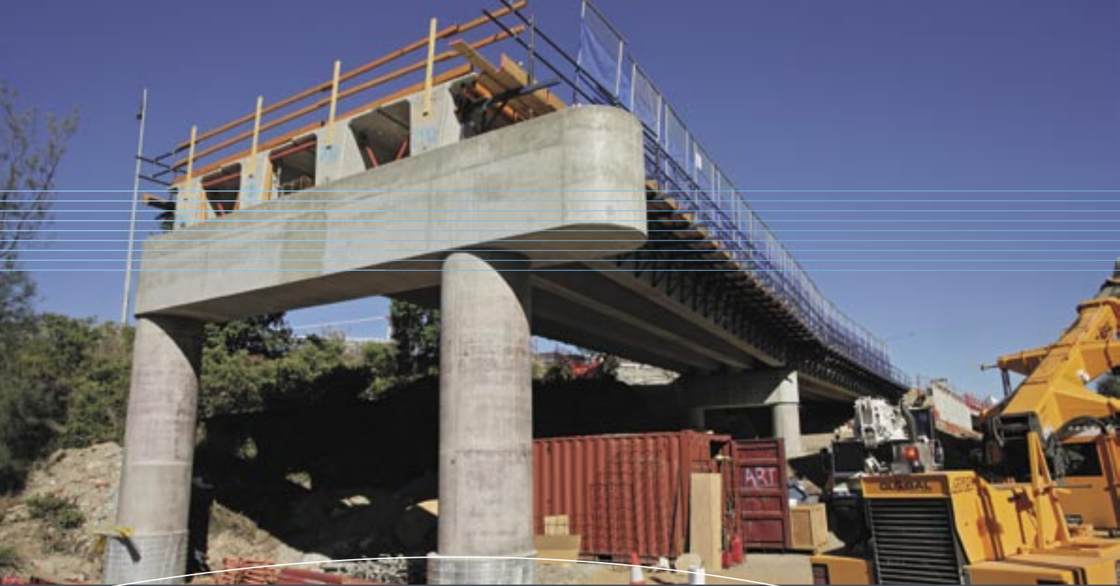
Bridge construction at Bowen Hills on the north side of the Brisbane River.
