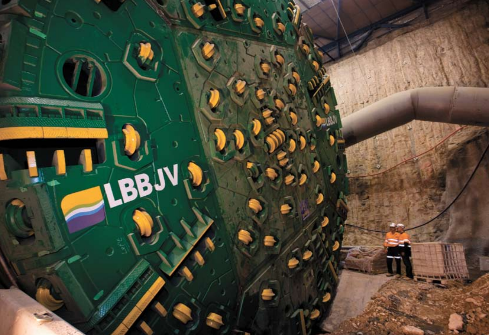
The second of two tunnel boring machines has started excavating rock and placing lining.
