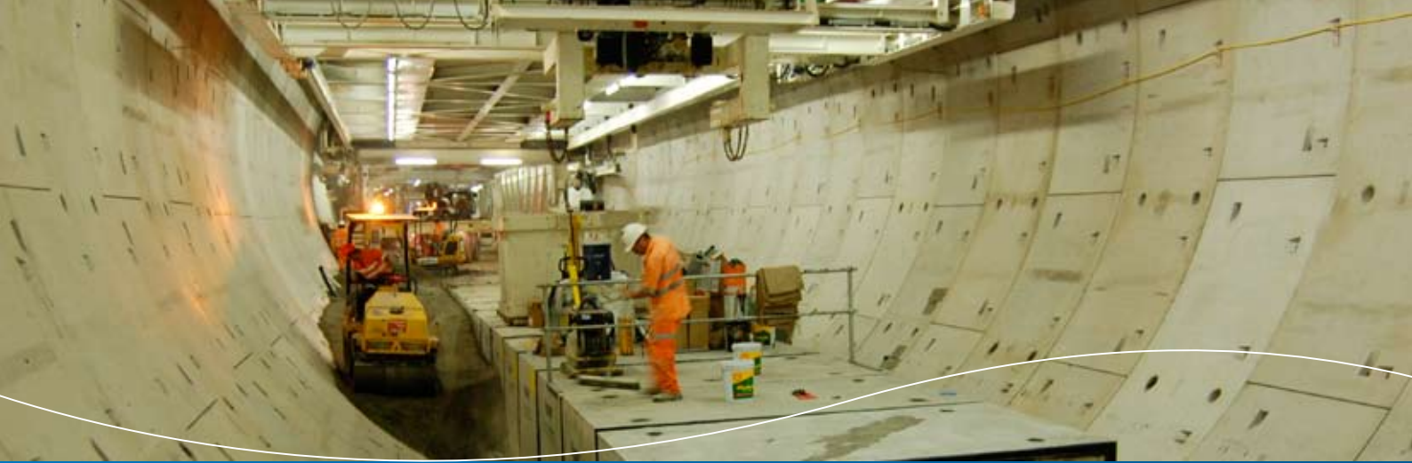
Tunnel workers install a 1.8 metre cable tunnel which will carry communication and other mechanical and electrical services below the road way.
